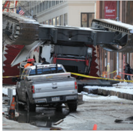
THE COLLAPSE of this crawler crane led City Hall to impose rules that have stalled projects.
